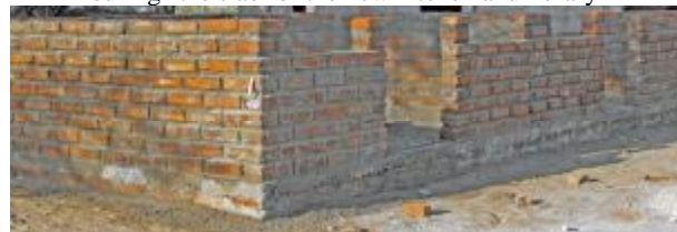
By the end of the month, we were half way up with the bricks!
